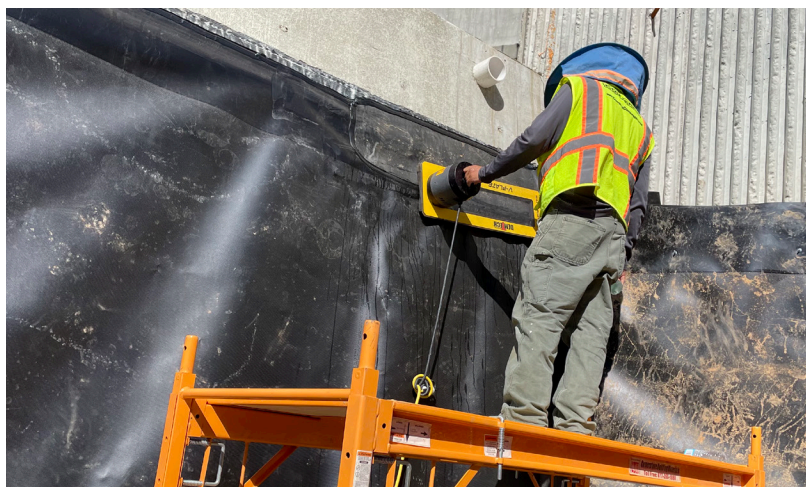
Work continues on the retaining wall support system on Jurupa Road at Van Buren Boulevard.
