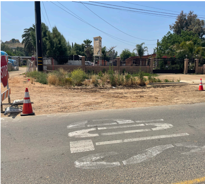
Crews will be installing improvements on the drainage system and working on utility relocation on Jurupa Road, see the photo above.
