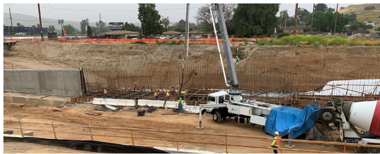
Crews placing concrete at the retaining wall system for the Jurupa Road underpass.
